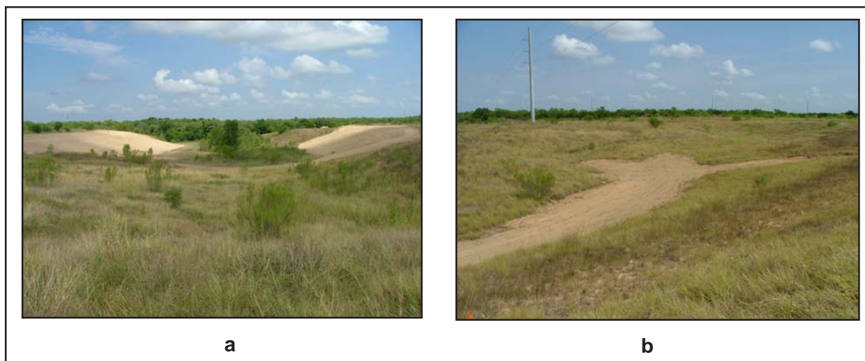
Figure 19. Photographs of the spillway trench after sloping and infilling in 2005: (a) the newly sloped north and south walls; and (b) the newly infilled gullies in the north basin.
