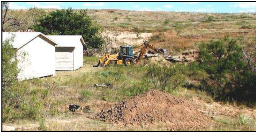
Figure 8-8. View of Southern Terrace Margin of Area B that Shows BT 24 During Excavation with BT 23 Backdirt in Foreground.
