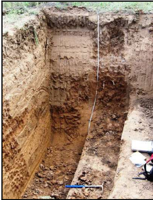
Figure 5-1. Example of Excavated Backhoe Trench (BT 6 east wall) with Safety Benches on Right Side.
